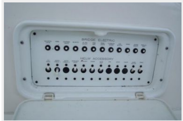
Flybridge Electrical Panel
