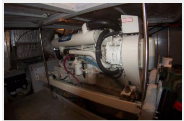
Starboard Cummins Diesel
