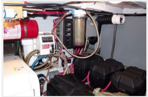
Oil Exchange System/Batteries
