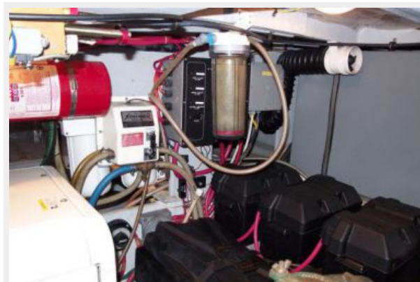
Oil Exchange System/Batteries
