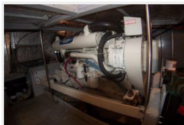
Starboard Cummins Diesel
