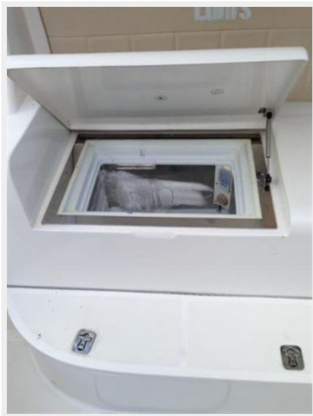
Freezer in Mezzanine
