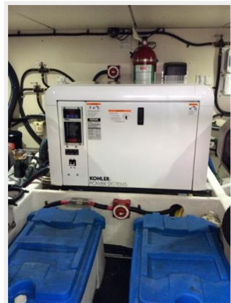
Kohler 10kw Generator
