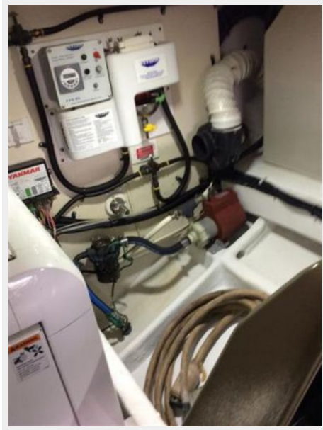
Fuel Polishing System Area in front of Stbd. Engine
