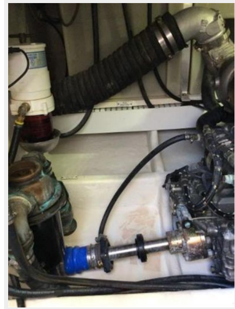
Port Shaft Log
