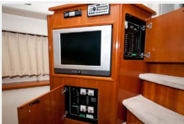
Salon TV and Electrical Panels
