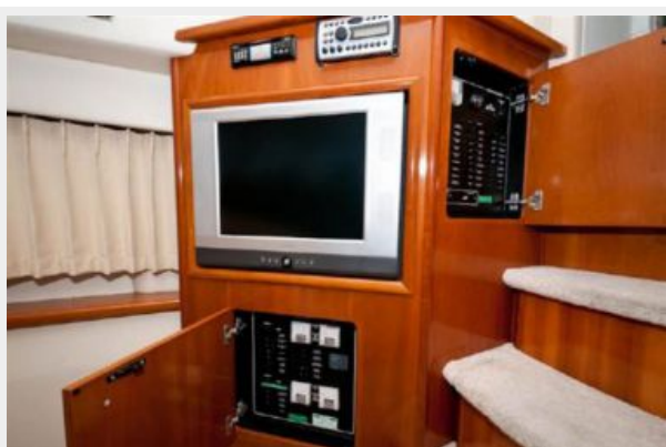
Salon TV and Electrical Panels
