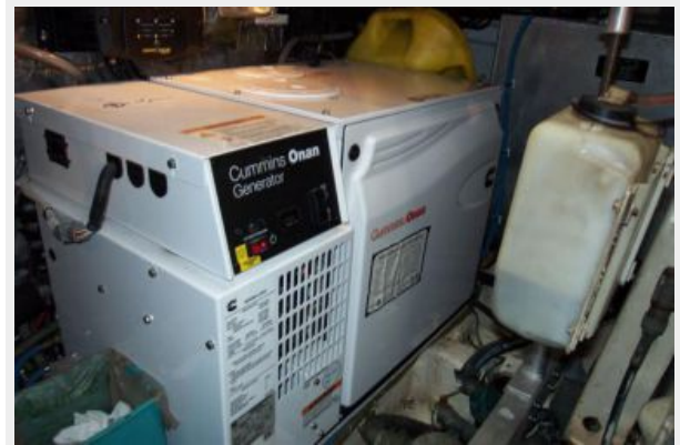
Cummins Onan Genset (New 2012)
