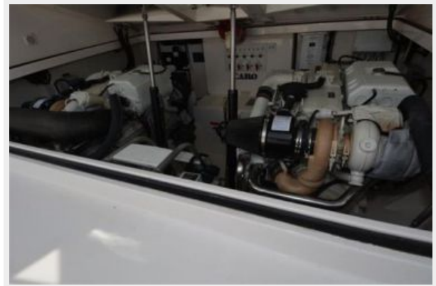
2005 Cabo Yachts 35 Express Engine Room
