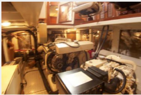
Clean Engine Room
