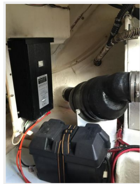
Engine Room View
