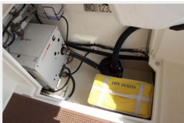
Onan 5 Kw Genset in Sound Enclosure
