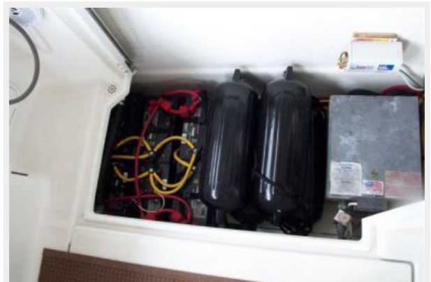
Battery Bank - Port Cockpit
