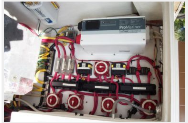
Charger/Inverter DC Switches, Water Heater
