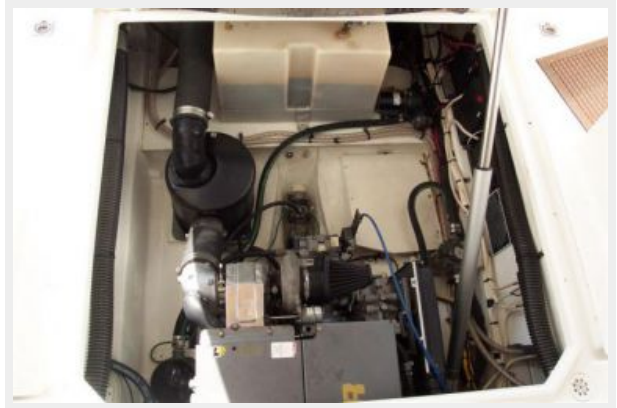
Yanmar - Clean Engine Room
