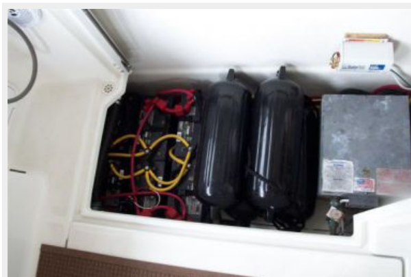
Battery Bank - Port Cockpit
