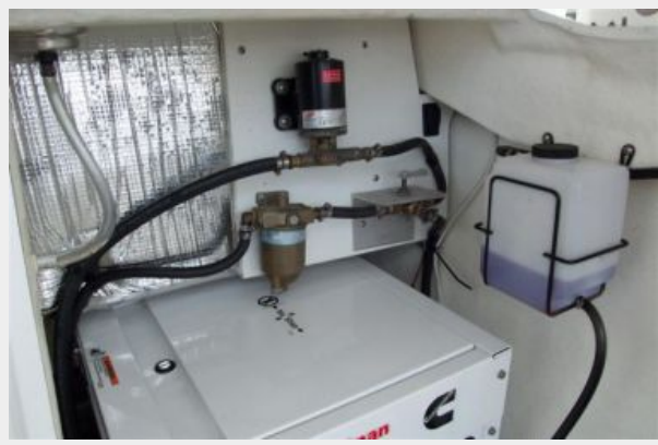
Fuel Transfer Pump
