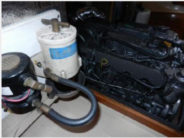
Starboard engine and filter access
