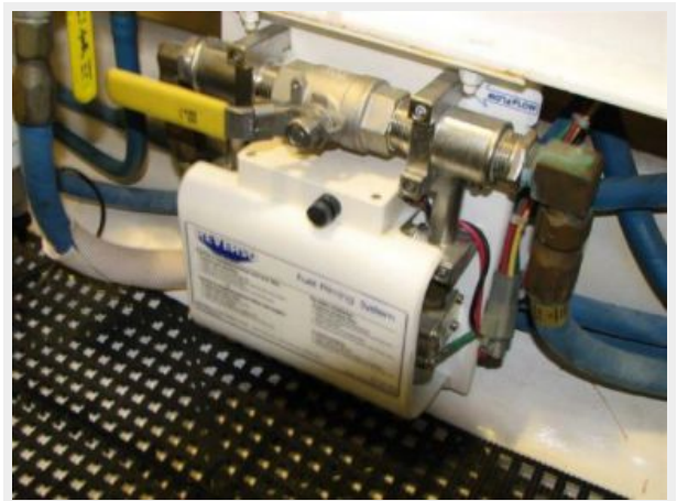
Engine & Mechanical Equipment 7 - Fuel Prime Pumps
