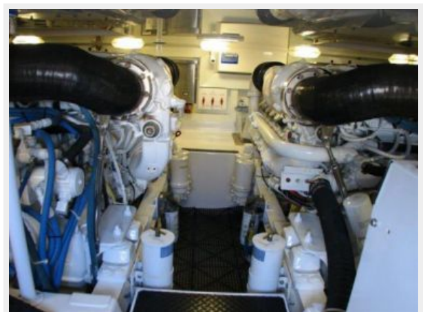
Engine & Mechanical Equipment 1 - Engine Room
