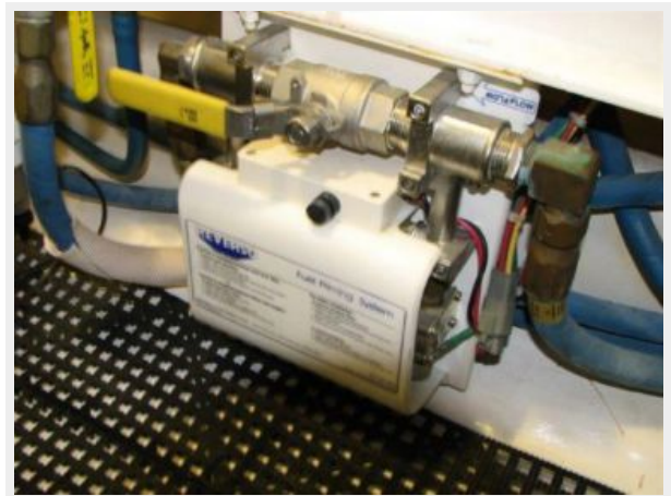
Engine & Mechanical Equipment 7 - Fuel Prime Pumps
