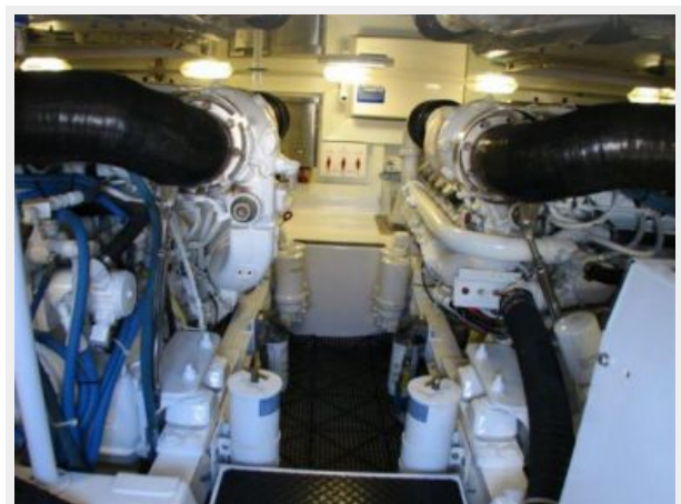
Engine & Mechanical Equipment 1 - Engine Room
