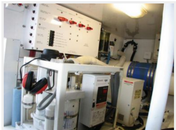
Engine & Mechanical Equipment 5 - Engine Room
