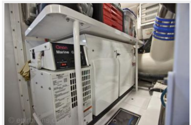
Port Onan Generator
