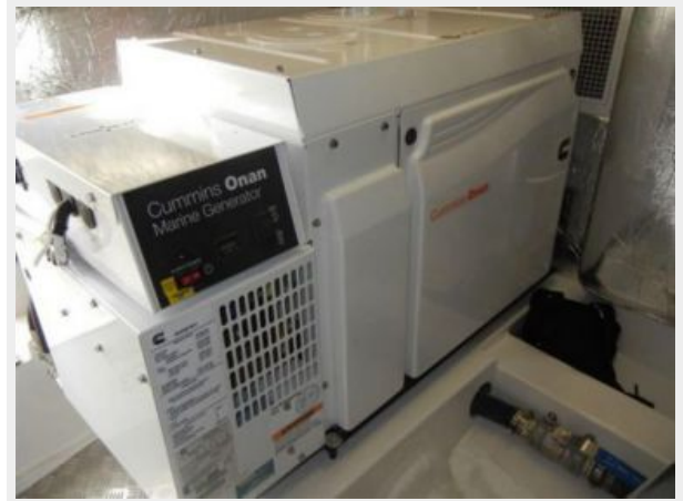
17.5 kW Onan Generator
