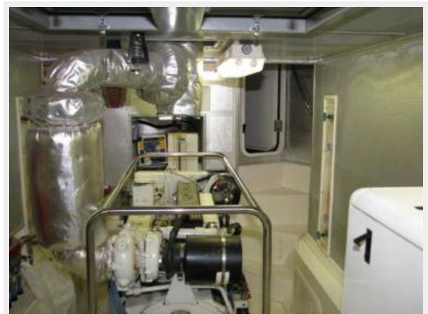
Engine room - main engine
