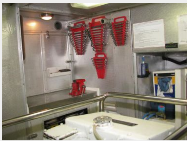
Engine room - forward
