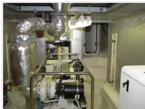
Engine room - main engine
