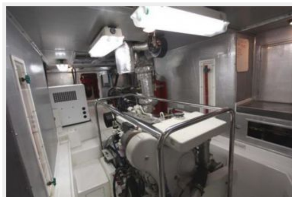
Engine room looking aft
