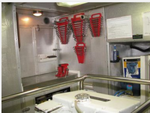
Engine room - forward
