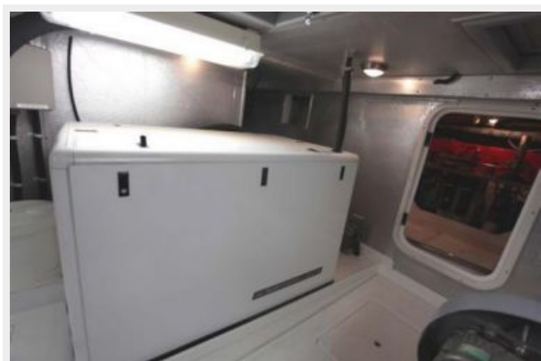
Engine room generator
