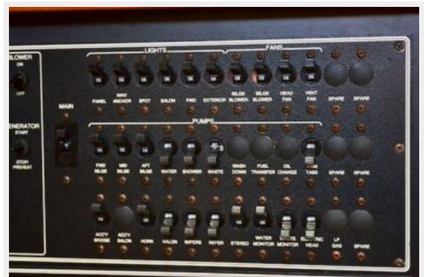
Main Distribution Panel
