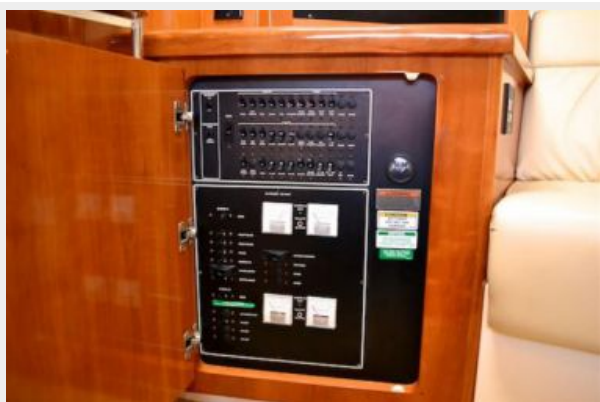
Salon Main Distribution Panel
