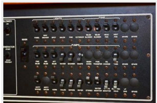
Main Distribution Panel
