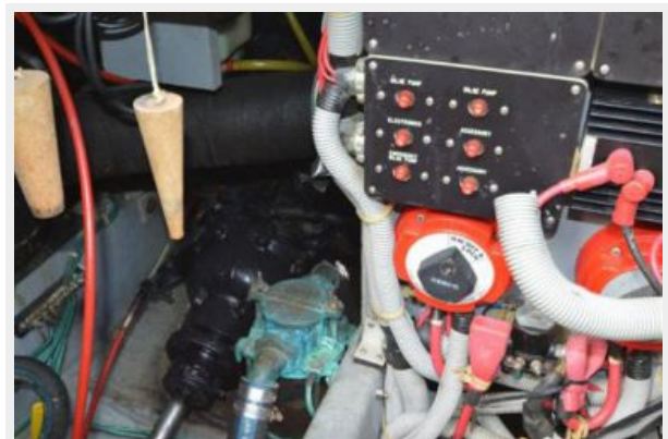
345 Sea Ray Sedan Bridge, battery switching
