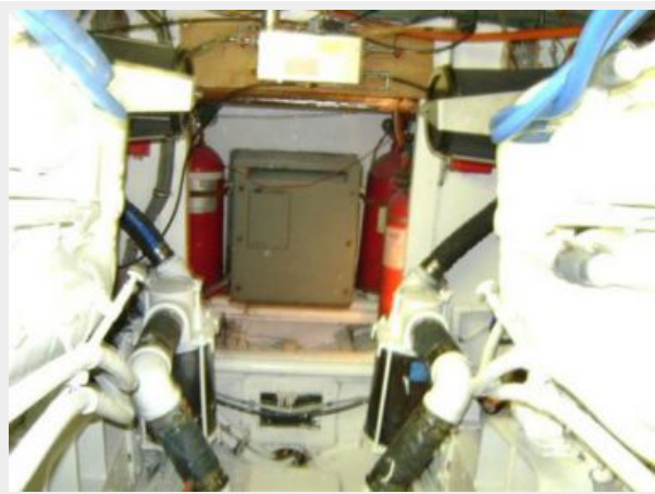
Main Engine Room
