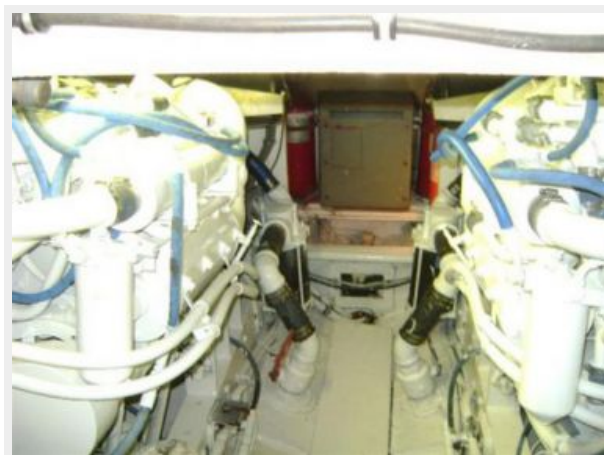
Main Engine Room
