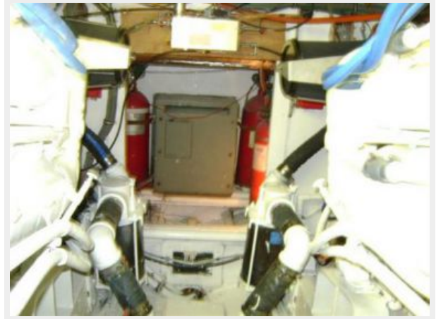
Main Engine Room
