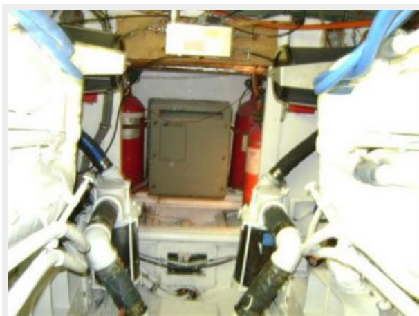
Main Engine Room
