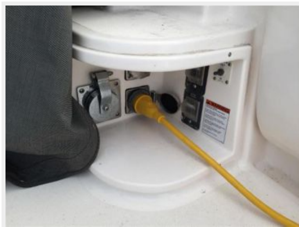
Starboard Shore Power Plug
