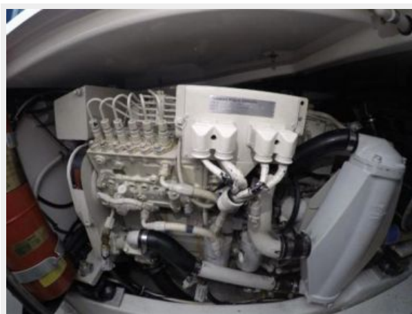
Starboard Main Engine
