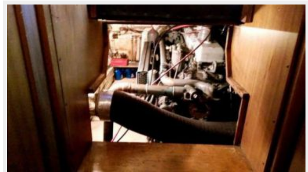
Engine Access from Aft Cabins
