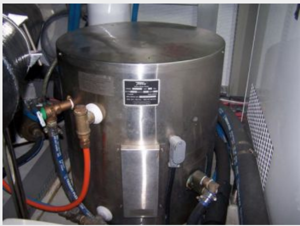
Hot Water Heater
