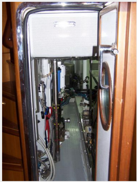
Entry Door to Engine Room
