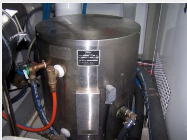
Hot Water Heater
