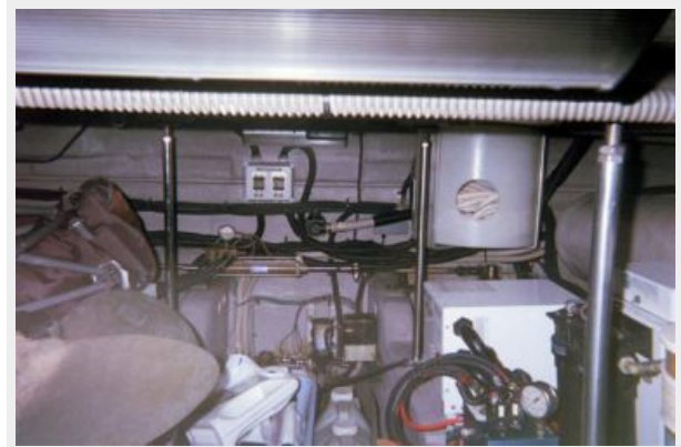
Aft System Compartment
