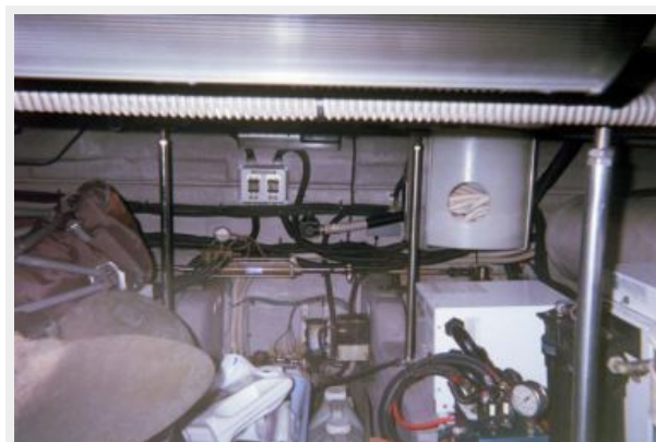
Aft System Compartment
