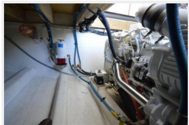
Outboard Access in Engine Room
