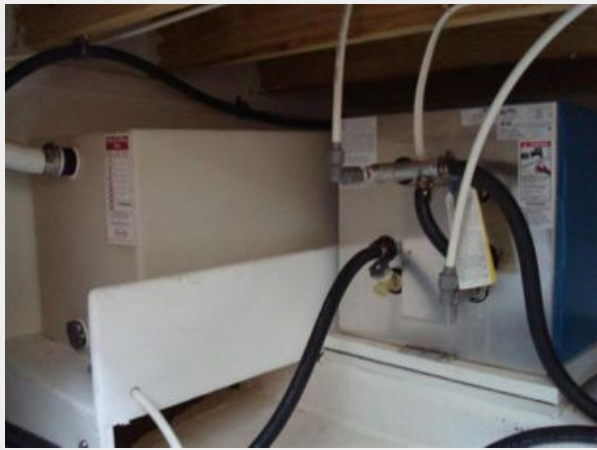
Freshwater Tank and Hot Water
