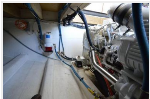
Outboard Access in Engine Room
