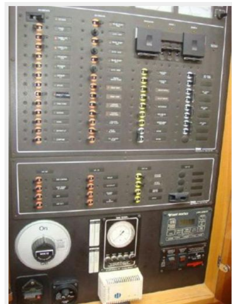
46' Alden electrical panel
