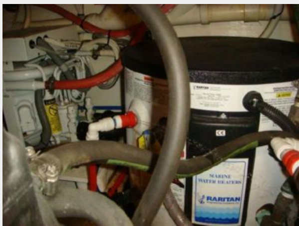
46' Alden water heater
