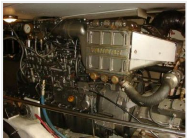
46' Alden starboard main engine
