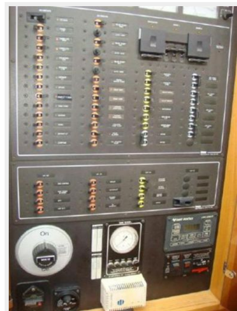
46' Alden electrical panel
