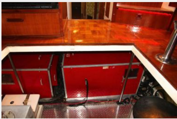
Genset with sound shield
