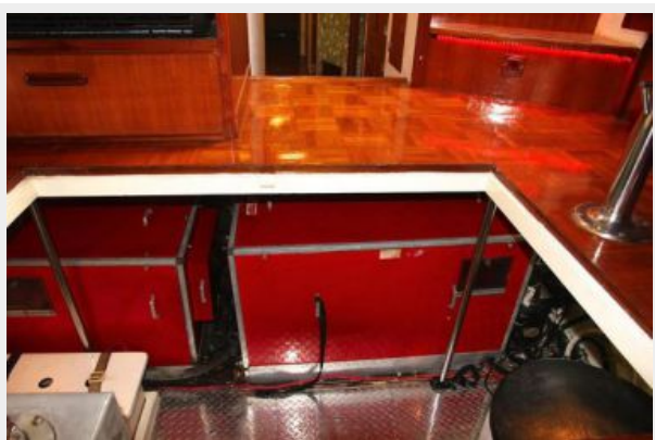
Genset with sound shield
