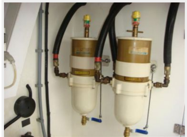
42' Sealine Racor fuel filters
