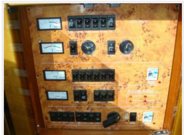
42' Sealine electrical panel
