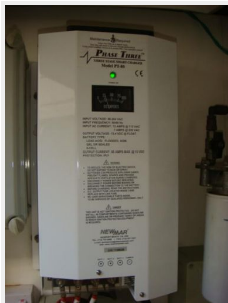
42' Sealine battery charger
