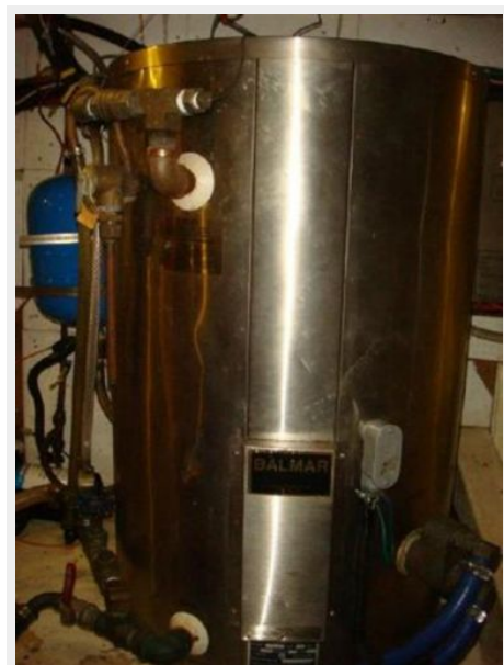
42' Kadey Krogen water heater
