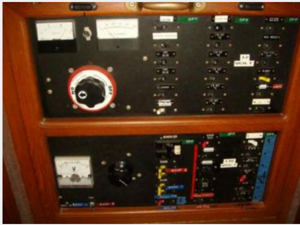
42' Kadey Krogen electrical panel
