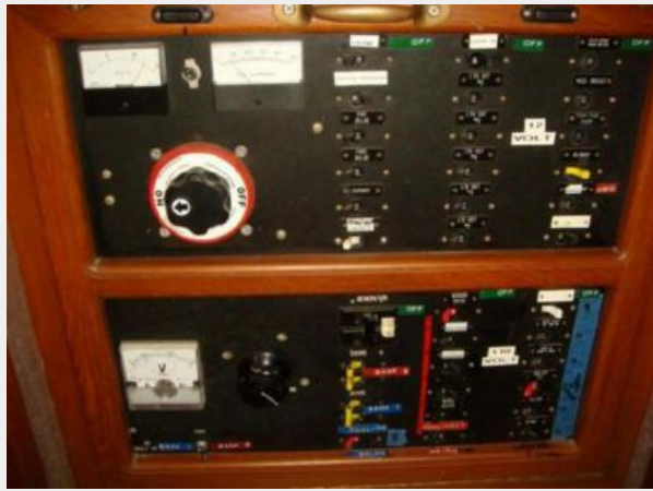
42' Kadey Krogen electrical panel
