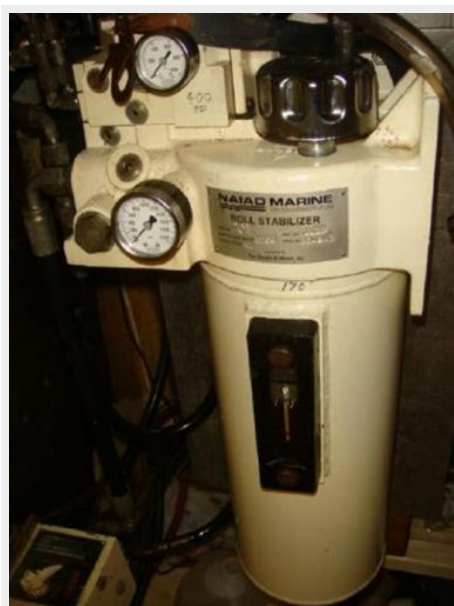
42' Kadey Krogen stabilizer system
