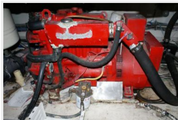
Westerbeke genset, 3069 hrs
