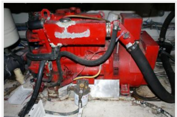
Westerbeke genset, 3069 hrs
