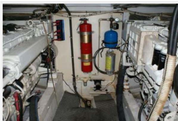
clean, organized engine room
