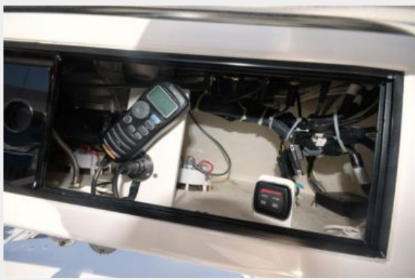
Tower Electronic Box
