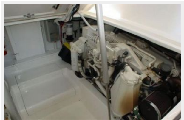
Starboard Main Engine
