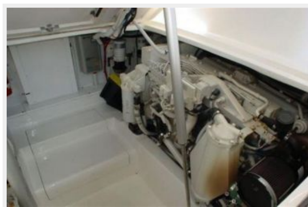
Starboard Main Engine
