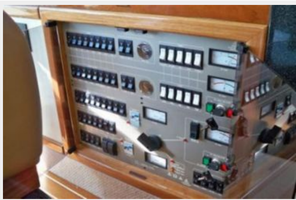
Main Distribution Panel
