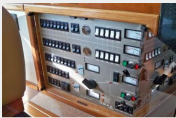
Main Distribution Panel
