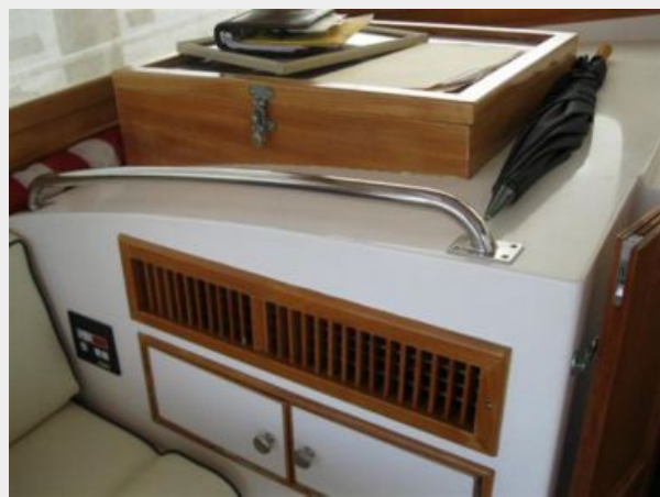
Cockpit air conditioning
